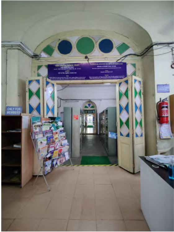
3. DOOR IN LIBRARY (D2 )
